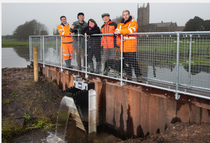
The tilting weir will help create a reliable feeding and breeding ground for birdlife
